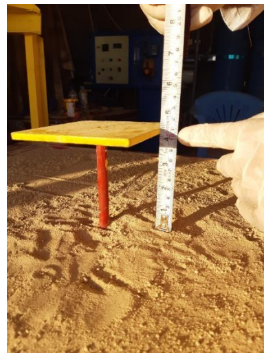
Figure 7. Gap between pile cap and soil surface.
